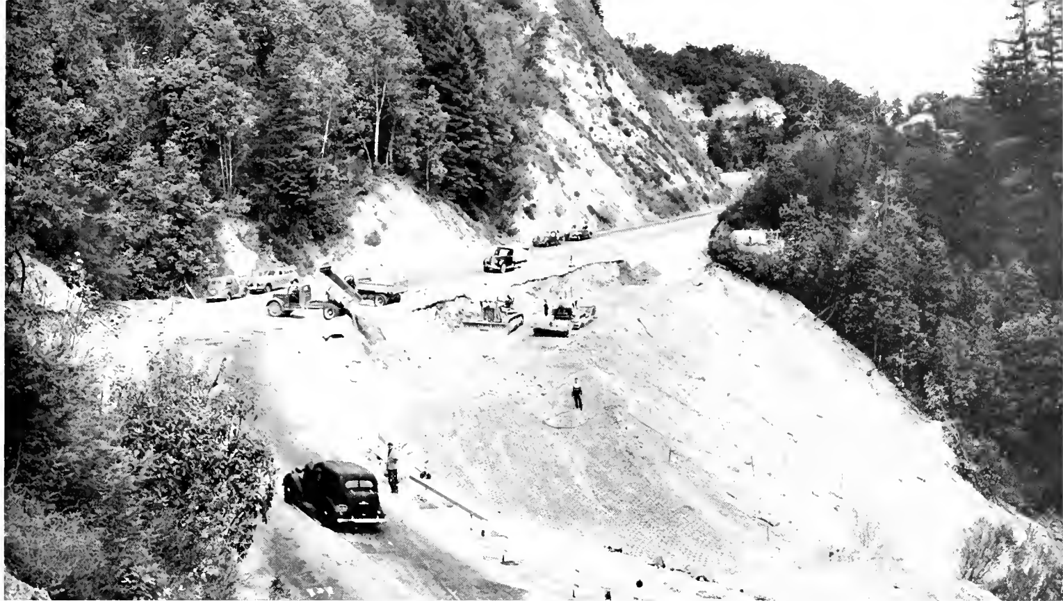
View of last stages of 30,000 cubic yard fill restoration at slipout on Los Gatos-Santa Cruz Highway.
